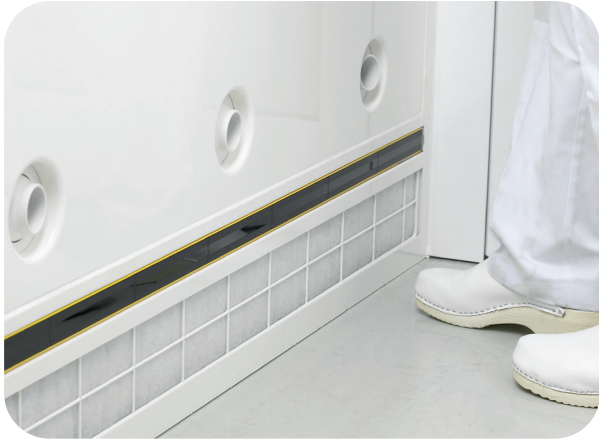
The lowest row of air nozzles is located close to the floor level for maximum efficiency.
